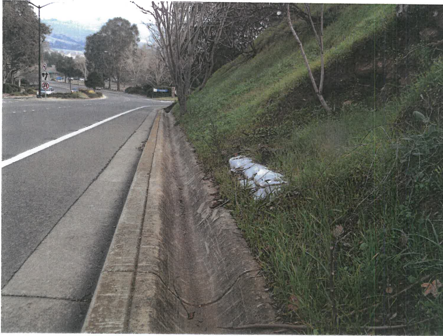
(#19) V-Ditch at the bottom of the hill.
