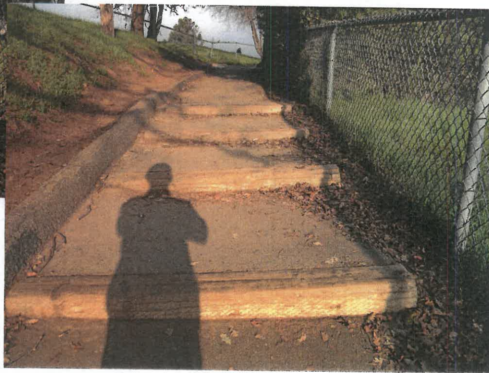
(#11) Steps on the uphill side of trail.
