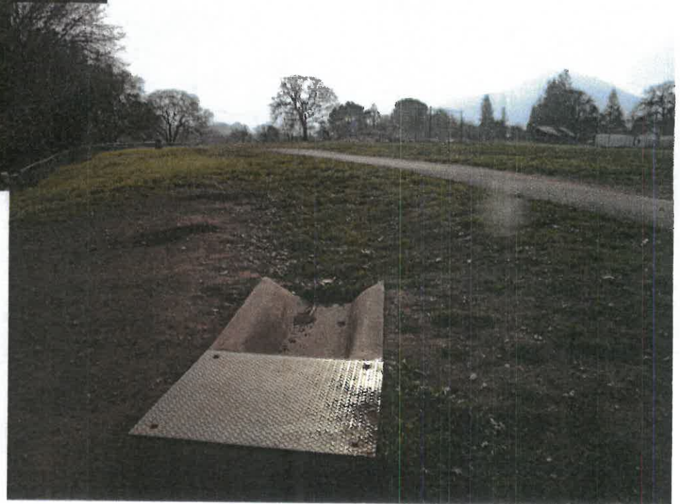
(#13) School property swale and drain.
