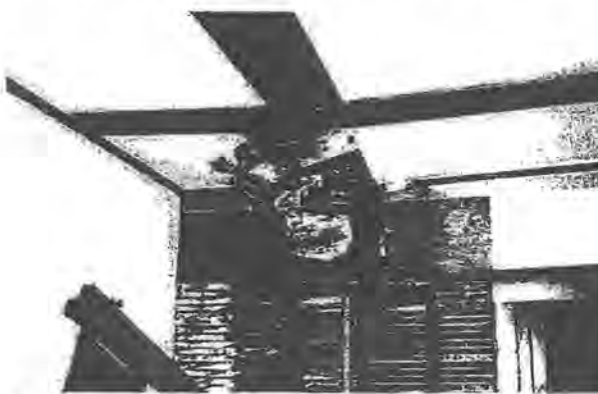
Water damage in Entry, facing east, 2001
