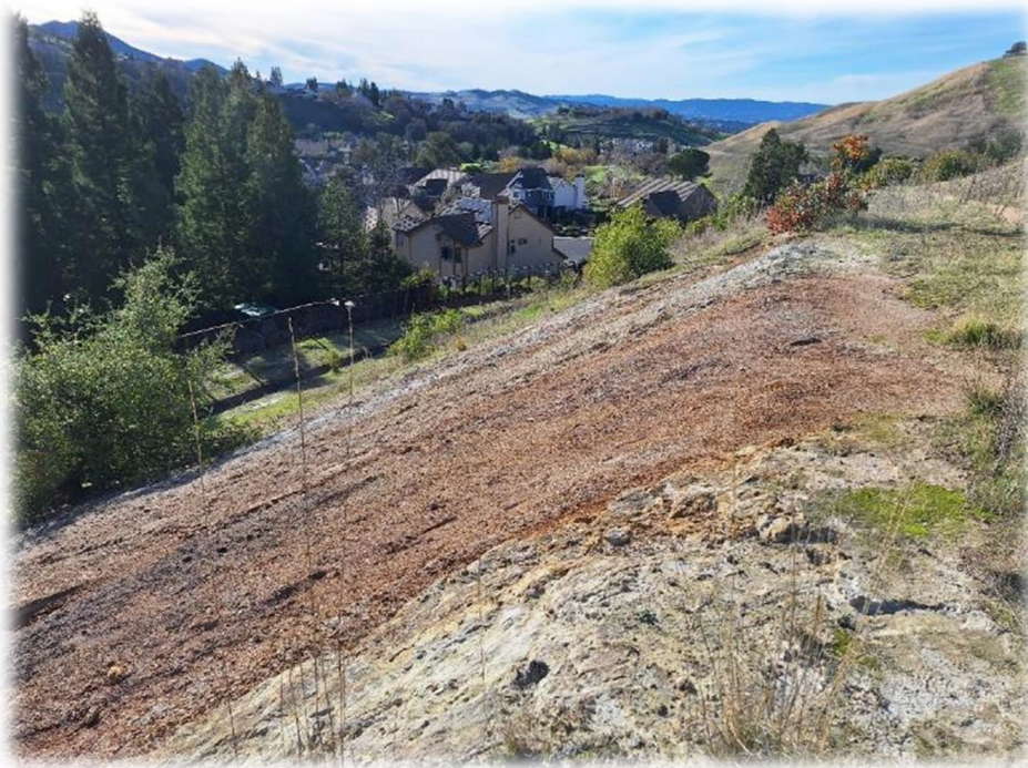
Photograph 3 – Additional slope erosion immediately south of Photograph 2.
